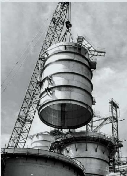
Safety at work had top priority in construction of the plant. There was also a separate safety procedure for crane work.
